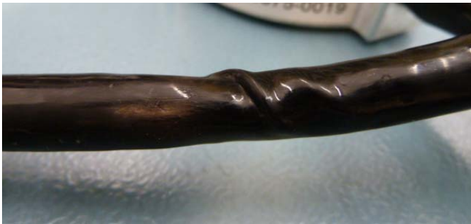
Figure 7: Damaged Motor Cable
