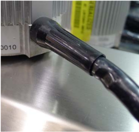
Figure 5: Cable Damage at the Motor Bend Relief
