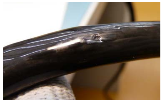
Figure 8: Damaged Motor Cable
