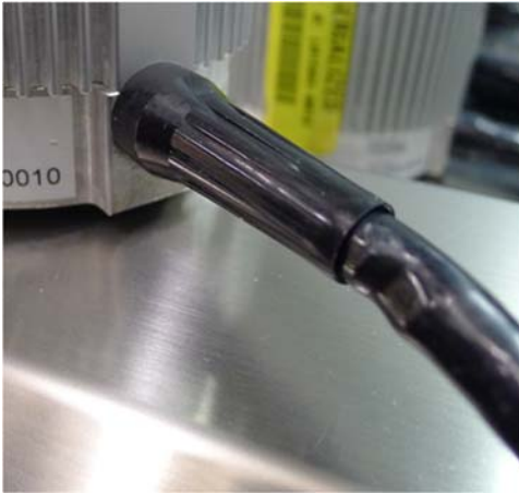
Figure 5: Cable Damage at the Motor Bend Relief
