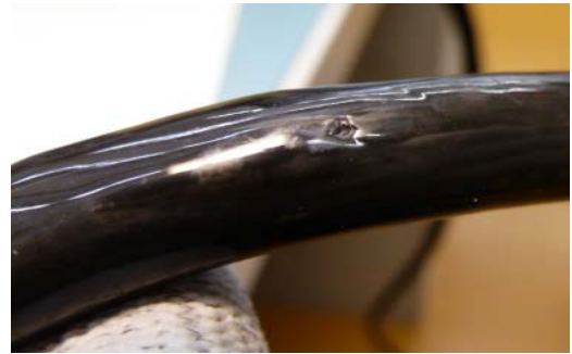
Figure 8: Damaged Motor Cable
