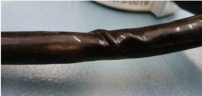
Figure 7: Damaged Motor Cable
